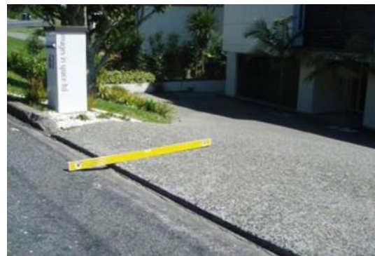
Figure 3: Poor vehicle crossing design
